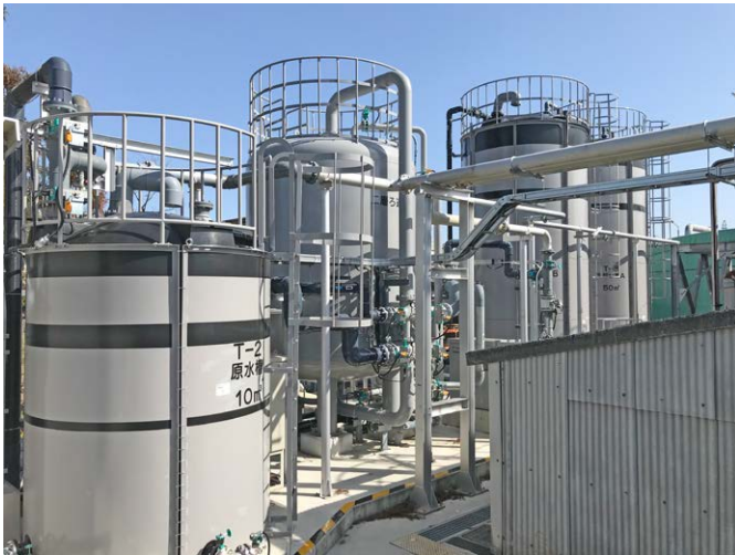
Water filtration equipment at the Shiga-Minakuchi Plant
